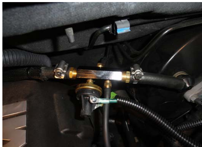
Vacuum Manifold Installed
