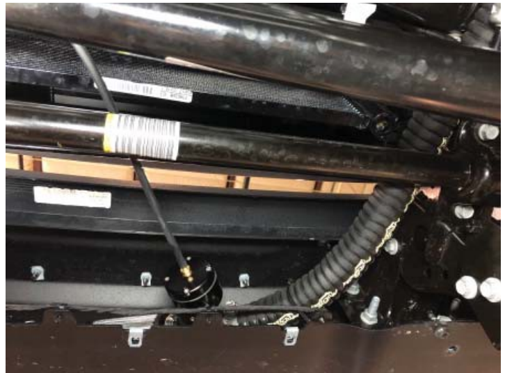
Surge Valve Installed
