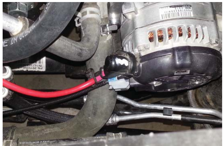
Plastic Cover Installed Over Power Wire
